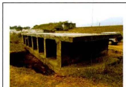
Photograph of incomplete culvert on road from Dimapur to Kujuni of Gosani Block under Gajapati District
