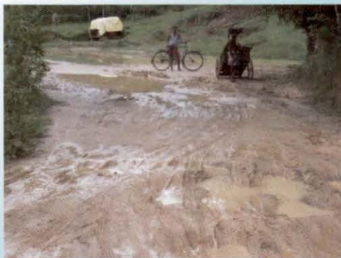
Road found full of mud and big potholes during construction period under package no. AS 13-59 in district Silchar, Assam
