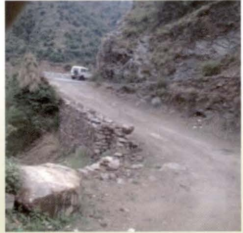
Road work from Chopda to Nalai, the quality of bituminous work was found poor at various places in Pauri district, Uttarakhand
