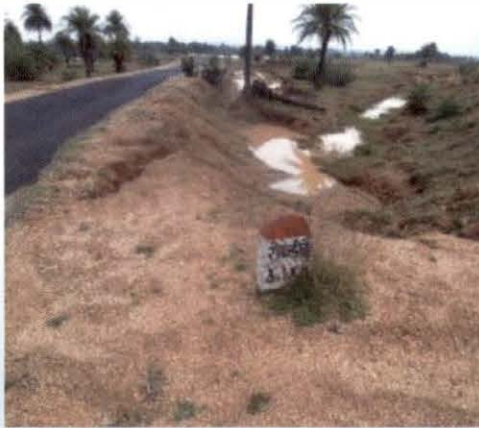
Road Raidih to Rajsar was completed without providing connectivity to Rajsar which was about 8 km. away from the end point of this road in Deoghar district, Jharkhand
