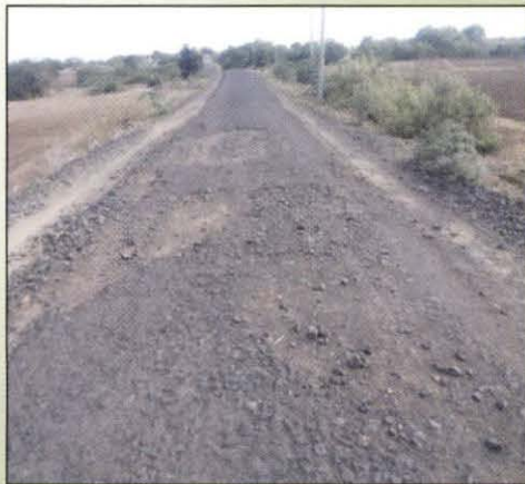
Deplorable condition of road 'KN 15-67-T-02 (Bankalga Cross) to Maharashtra Border' at Afzalpur Taluk in Kalaburgi district, Karnataka
