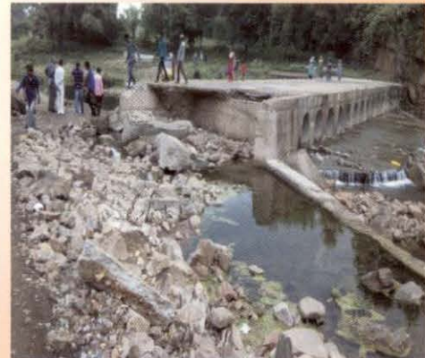
Part of vented culvert at the chainage 1/800 of road 'Kamboi Patel falia' washed away due to non-construction of pipes to allow the water to cross safely in Dahod district, Gujarat
