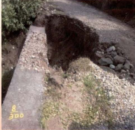
Non- construction of adequate number of cross drainage and poor construction in road Galak to Upper Rajwalta in Kathua district, Jammu and Kashmir
