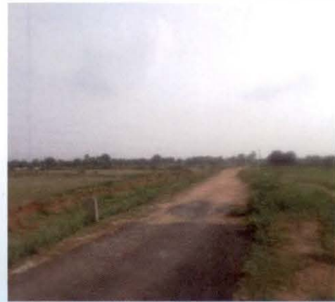
Unconstructed portion of road (more than 500m) left the habitation as unconnected (in L046 to Jala, Block Garhwa Hazaribag district, Jharkhand)
