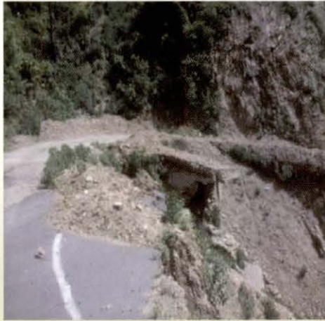
Road Naugaon-Bhukhandi was found damaged in Pauri district, Uttarakhand
