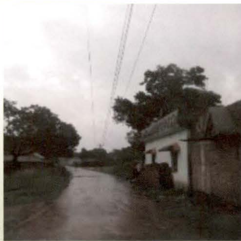
Non-construction of side drain in Baidynathpur to Bahadurpur in Deoghar district, Jharkhand
