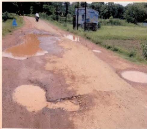
Potholes developed on Marthapur-Jamunakote road due to non-maintenance of road Dhenkanal district, Odisha
