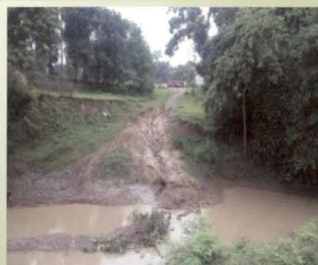
Cross drainage work not executed (Road work 'T02 KULI KUKDA - BASAHA (package CG 0268)' in Bilaspur district, Chhattisgarh)
