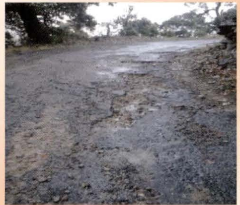
Bituminous work of road Mailsain to Chopda was found damaged at various places in Pauri district, Uttarakhand
