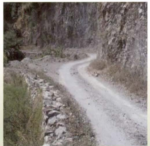
Poor quality of road construction in Bhorsa-Pinro, Nainital district, Uttarakhand
