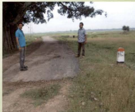
Dead end of road not constructed (Road from 'Chanchaki to K.A. Road- in Assam, HPIU, Nagaon Road Circle, Nagaon- AS 19-246).
