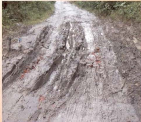
Deplorable condition of road 'Baraigram to Pecharpar', AS 13-36 due to non-maintenance in, Karimganj district, Assam
