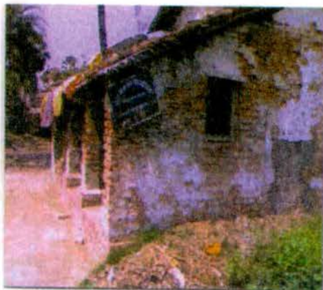
Unsafe and dilapidated Anganwadi Centre at Dhuiya Tola under Cheria Bariyarpur Project, Begusarai
