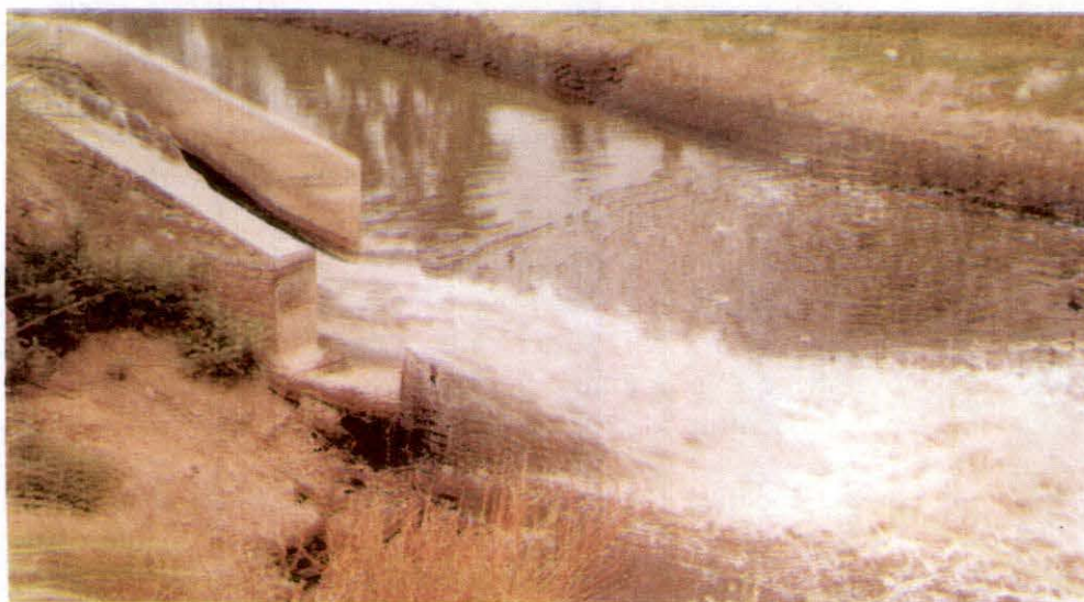
Treated effluent from 25 MLD, STP at Camp area Yamunanagar coming out through effluent channel and falling into a Nallah running near the STP which flows into WJC
