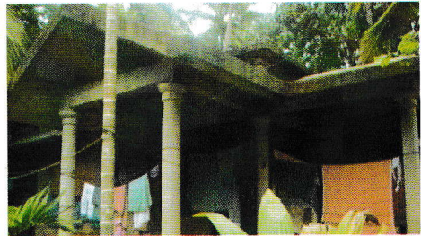
An unfinished house which did not adhere to plinth area limitation
