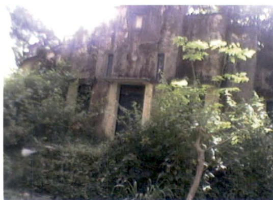
SISI building in dilapidated condition
