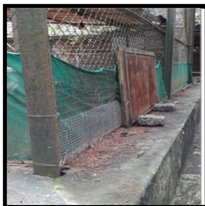
Pic.7: Temporary measure to cover damaged enclosure (Picture taken on 28 September 2017)
