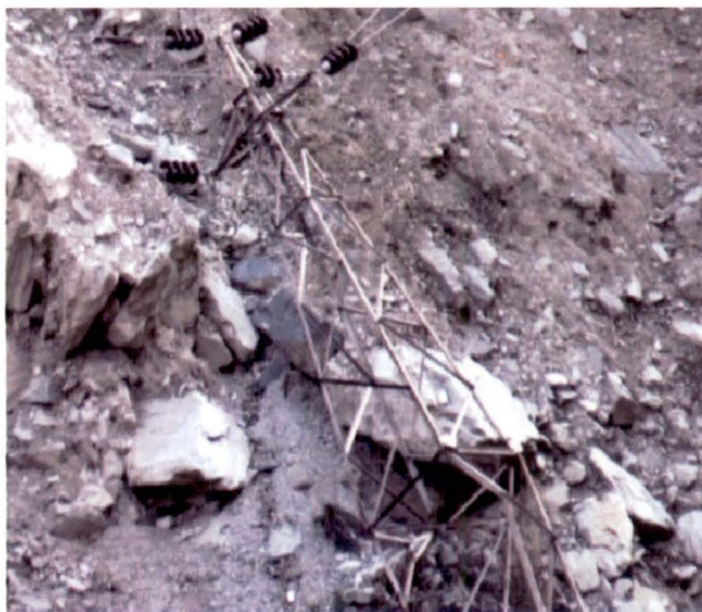
Unrestored electricity transmission line at Khet (Pithoragarh) 03.01.2015
