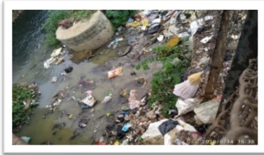
Sewage flowing in SWD at Ejipura, Koramangala Zone
