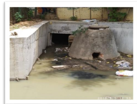
Discharge of sewage into SWD through fractured manhole at Seshadripuram, West Zone
