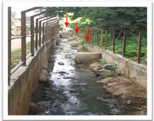
Sewage flowing in the SWDs due to chain of fractured manholes in the drain connecting to Herohalli Lake, Dasarahalli Zone
