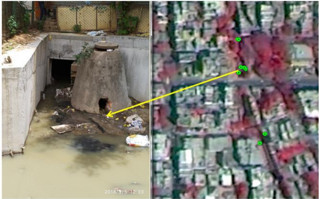
Discharge of sewage into SWD through fractured manhole
