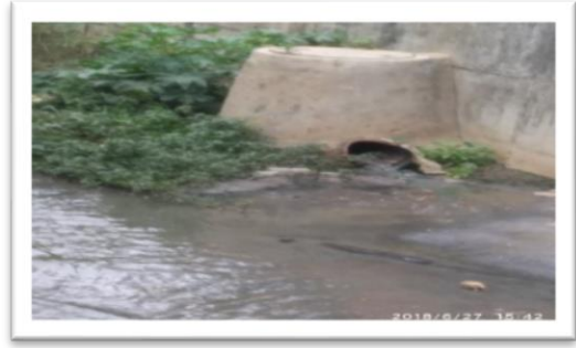
Discharge of sewage into SWD through fractured manhole at Yeshwanthpur, RR Nagar Zone
