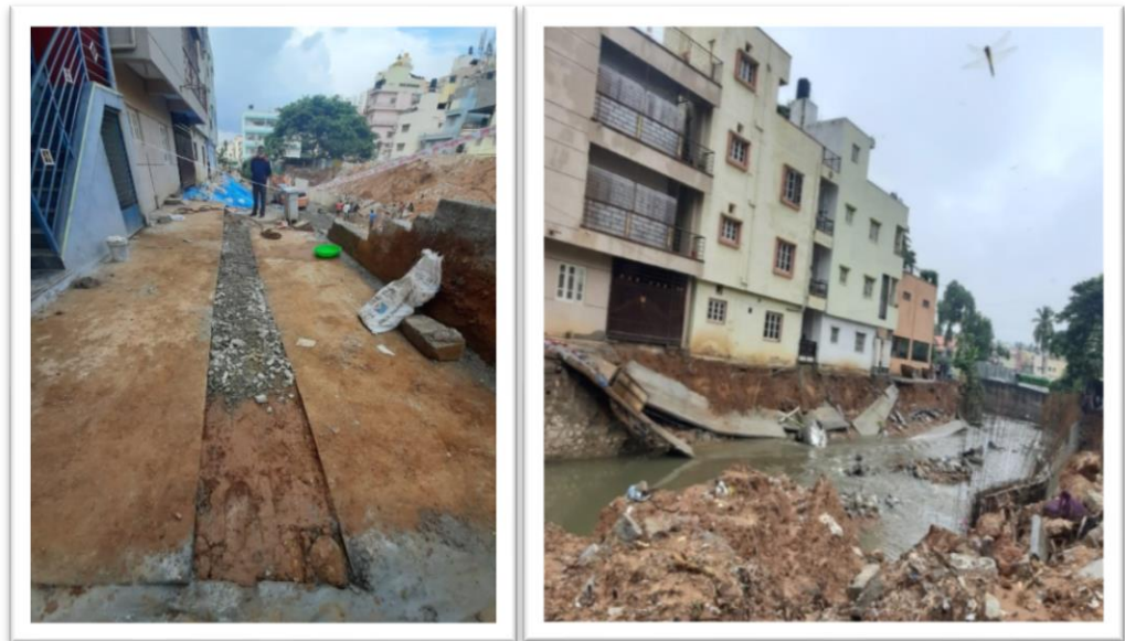
Exhibit 3.1: Damage to SWD retention wall and concrete road
