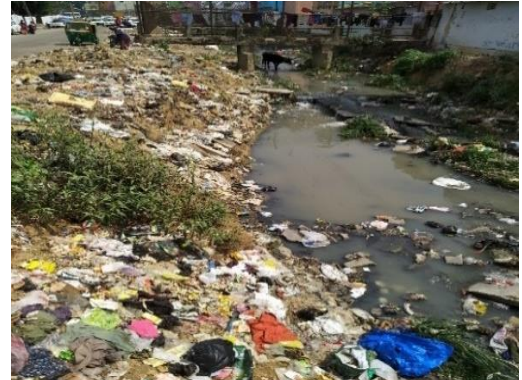
Dumped debris/wastes and garbage inside SWD at Ejipura, Koramangala Zone
