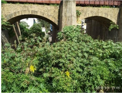
Vegetation inside SWD at Magadi Road Railway Bridge, West Zone
