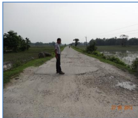
Dilapidated condition of Topia to Balijuri Road- Package No. AS-22-27 (27-05-2012)
