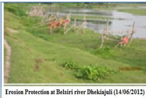
Erosion Protection at Naharbari-Dhekiajuli Block (14/06/2012)
