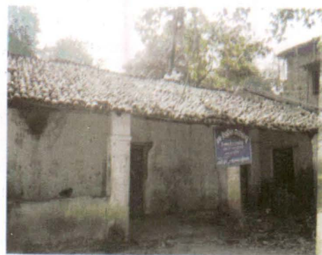
Dilapidated office building of the Gudighat watershed in Muribahal Block (Bolangir district)
