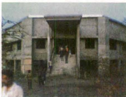
Incomplete community hall building at VRC land at Nagpur
