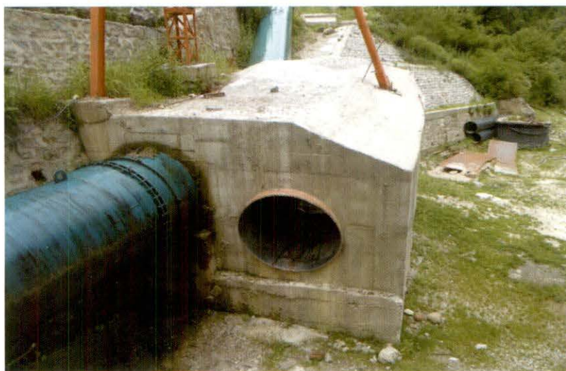
(Penstock of 5MW Toss Hydro Electric Project with scope for 20 MW)
