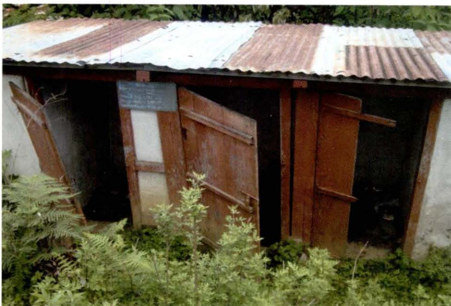
Deteriorated School Toilet at Sange, Dirang, West Kameng district !
