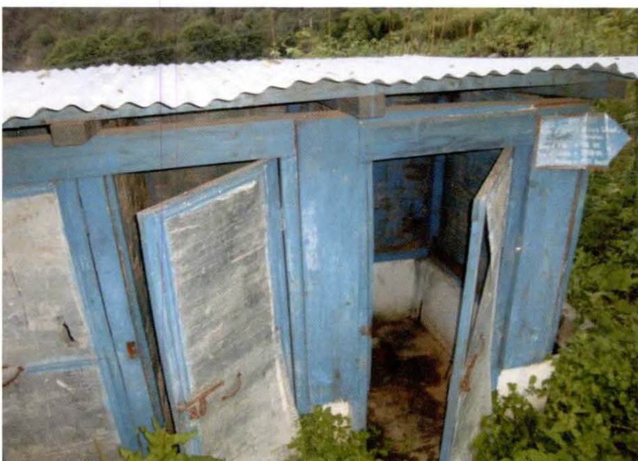
Deteriorated School Toilet at Wanghoo, Singchung Block, West Kameng district !
