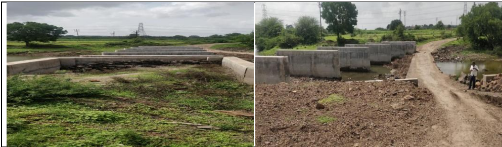
Incomplete approaches and deck slab of Nilwandi Bridge due to fund shortage
