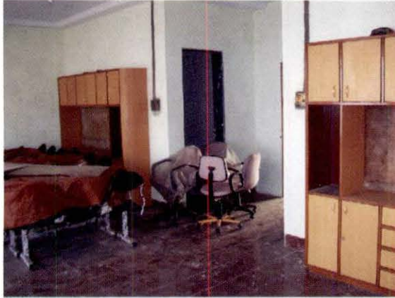
Office for MMB in Mandwa Terminus Building constructed out of IWT funds
