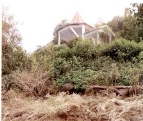
Approach to Passenger Shed at Nakranaghat not constructed
