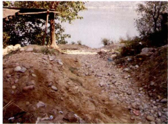
Jetty at Jeoripattan not constructed
