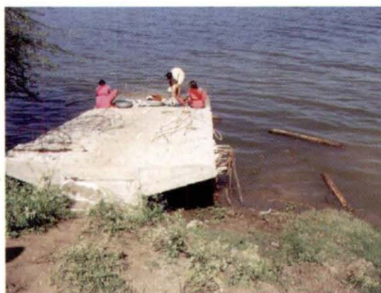
Lack of approach road for jetty at Mohanpur
