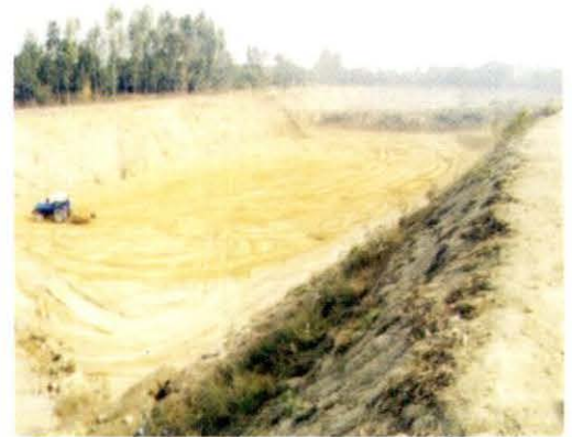
Development of site for Cell No.3 of CHWDF at Leather Cluster, Kanpur
