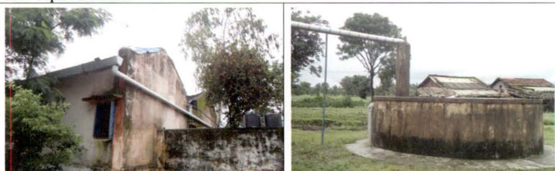
Roof top water harvesting and RCC surface tank for collection of roof top water at a cost of ₹ 4.38 lakh, completed in February 2012 at Pre-Matric Tribal boys Hostel having capacity of 50 boys, at village Khedi Sawligarh, Betul block of Betul District.
