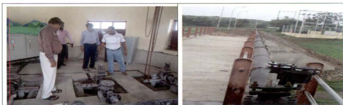
Intake well-cum-pump house and approach bridge to the intake well, installed pipe line, air valve and sluice valve installed at Village Velgipada, Sardarpur in Dhar district for covering 44 habitations in Badnawar/Sardarpur blocks of Dhar district for pumping raw water to the treatment plant, the work was completed in March 2013. After testing, water is being supplied since September 2013.
