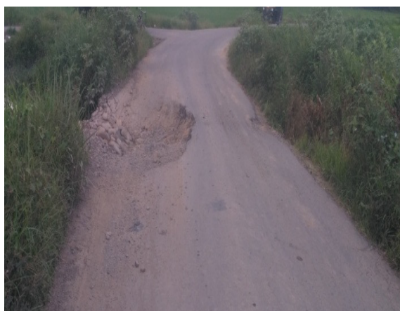
Improvement of Lamsang Sekmai Road (Badly damaged portion) (16 August 2018)
