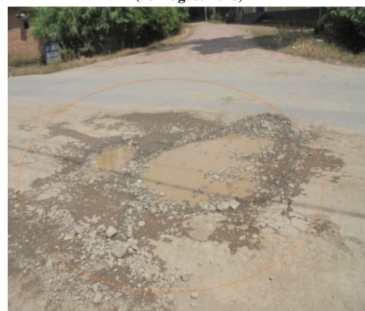
Improvement of Thoubal Charangpat Road via Nepra Company (Pothole at RD 7.8 km) (20 August 2018)
