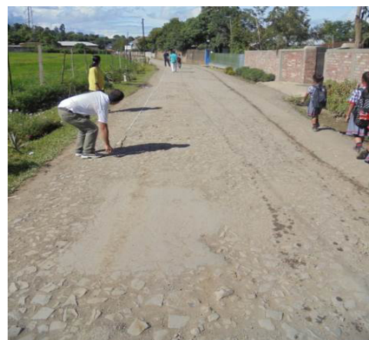
Improvement of Roads in and around Churachandpur District Hqrs (Worn out bituminous surface for a length of 200m at Marian street) (28 August 2018)
