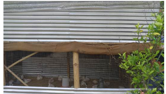
Structure constructed was being used as poultry house at the time of Joint Physical Verification. (28 March 2019)
