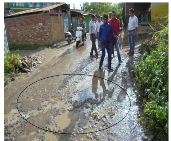
"Improvement of M.I. Bishnupur road and M.I. Bengoon" (Badly damaged portion of the work 'School Leirak, Ningthemcha Karong Road') (6 June 2018)
