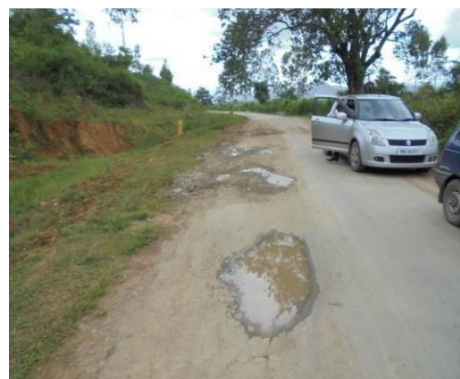
Poor condition of road near Benggi (20 August 2018)
