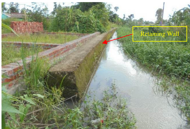
Retaining wall constructed downstream at Bisnunaha was not connected with the bridge and started from 100 m away from the bridge downstream (20 August 2018)
