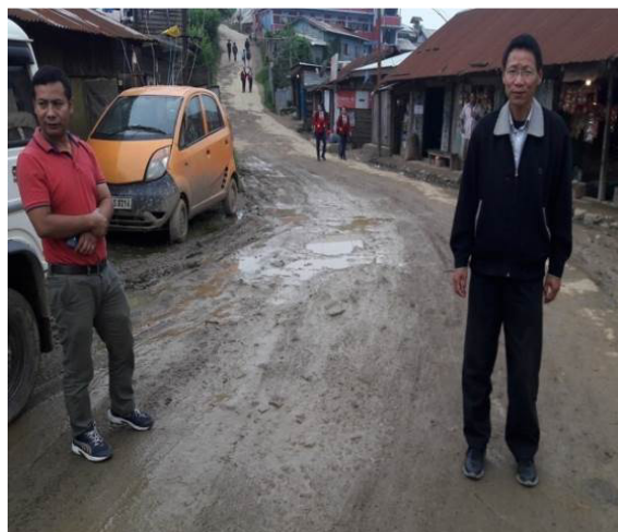
Improvement of Ukhrul District Hqrs road ( Damaged portion of Approach road to District Hospital) (12 July 2018)
