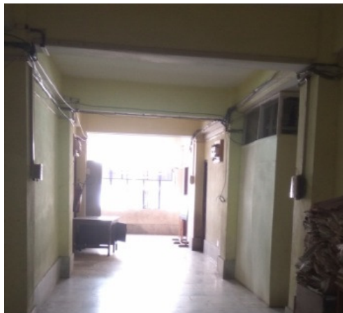
DMIS office with no CCTV camera, fire extinguishers, smoke sensors etc. (19 September 2018)
