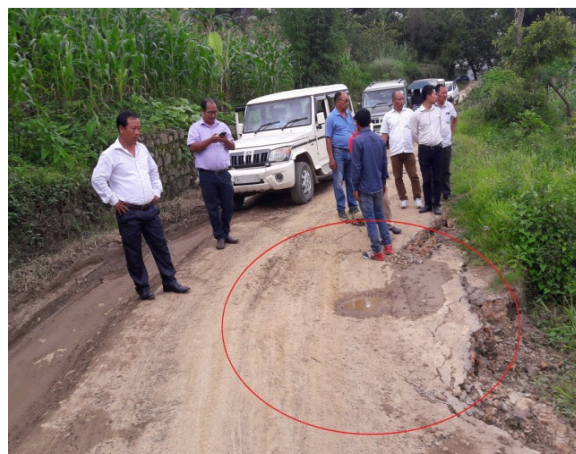
Sunken portion of 'Senapati Hqrs. Roads (Colony road) (30 June 2018)
