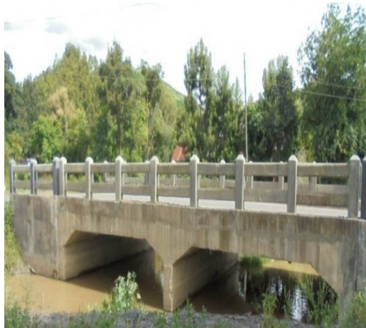
Bridge at Khoirom constructed under Asian Development Bank funding where the bridge under RIDF had again been proposed (20 August 2018)
