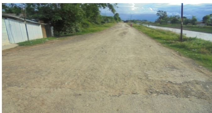
Unsurfaced road stretch of Wangjing Tentha Road-RD 7.6 km to RD10 km (20 August 2018)
