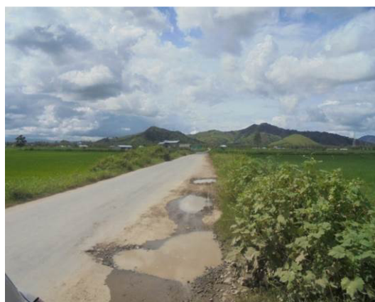
Poor condition of road at RD 2 km (20 August 2018)
