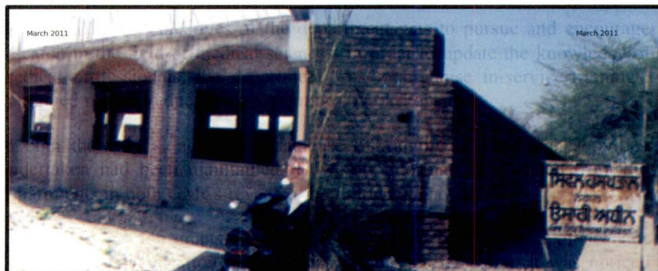
Incomplete building of Hospital at Nangal
