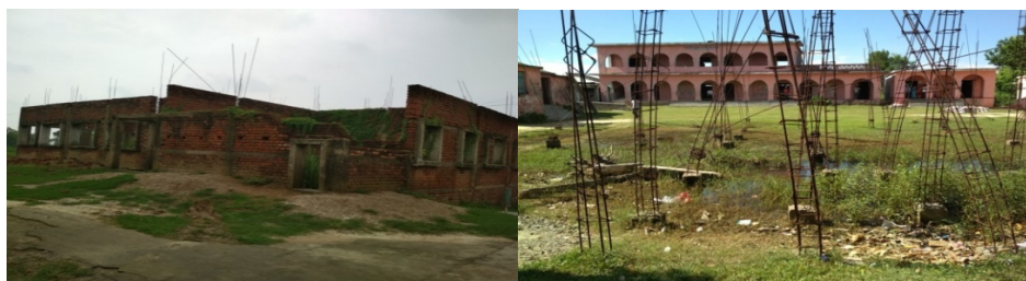
Upgraded Secondary School, Devchanda, Middle School, Andharvan, Madhubani Piro (USS-6, photo dated 11-07-17) (SSS-199, photo dated 20-07-17)
