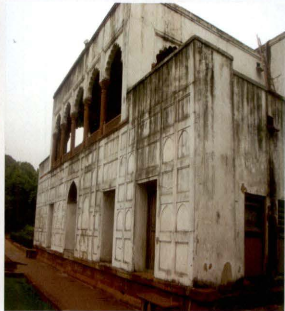
Rear of Diwan-e-Aam in need of chemical cleaning
