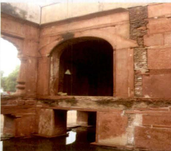
Missing stones and water logging in Jahaz Mahal
