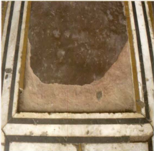
Broken flooring of the mosque
