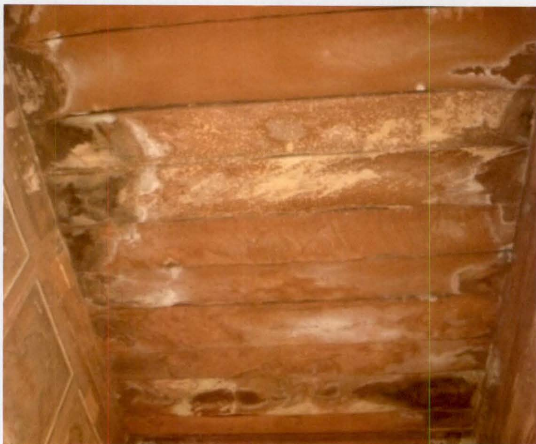
Seepage on the roof
