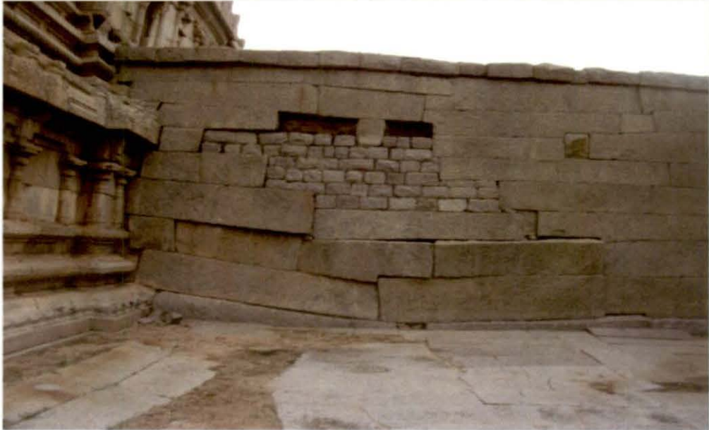
Cracks in Krishna Temple, Hampi, Bengaluru Circle
