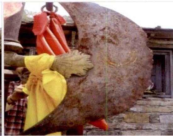
Rusting on part of a monument
