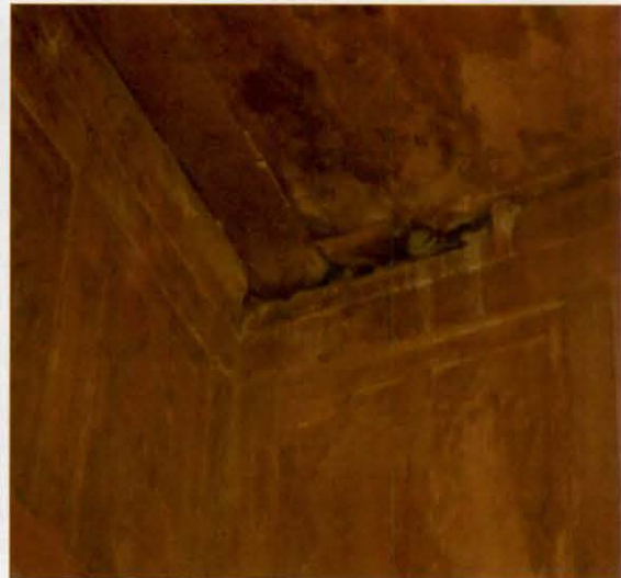
Seepage and cracks in the Mehman Khana
