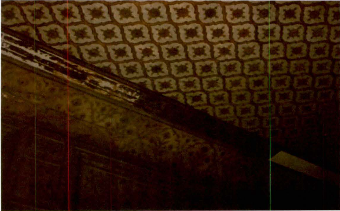
Missing design on the wall
