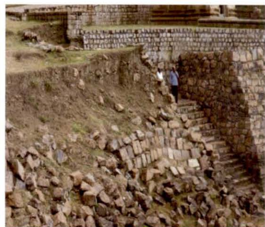
Chinnakavandanur, Sangagiri - Damaged side wall of the lower tank
