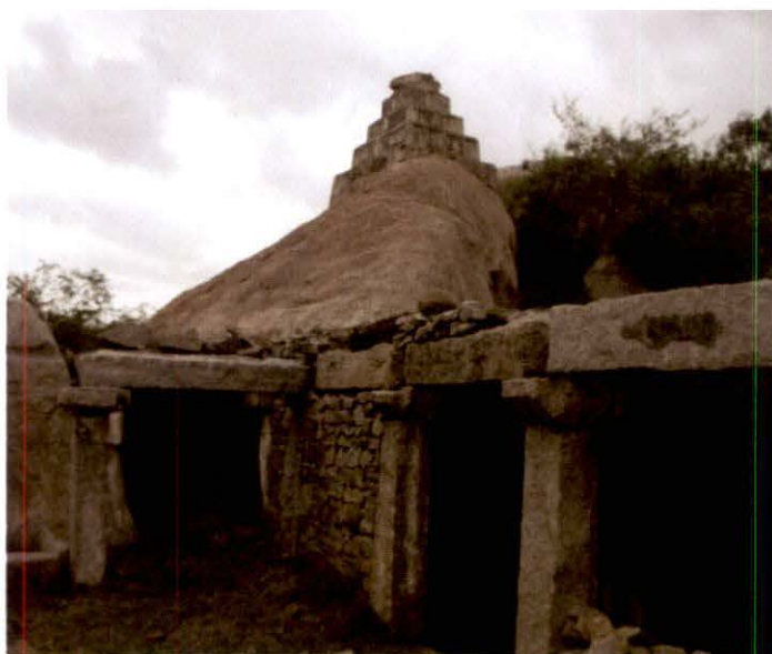
Dilapidated condition of the Saraswathi Temple, Bengaluru Circle
