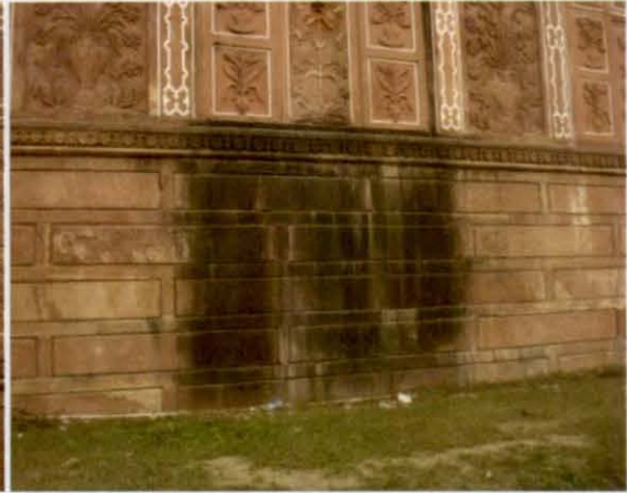
Stains on the stone
