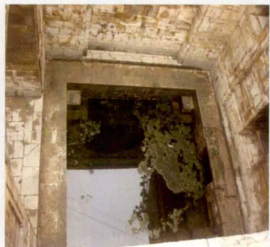
Stagnant water in Baoli
