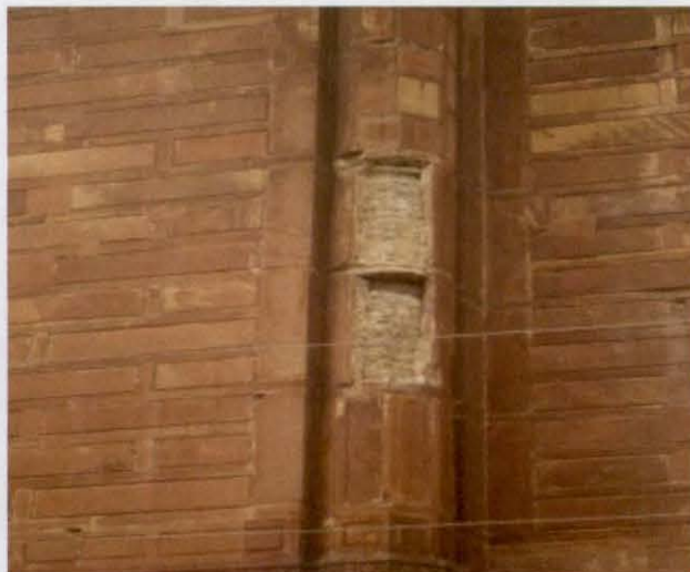
Missing stone and plaster
