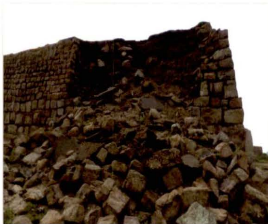
Chinnakavandanur, Sangagiri – Fort bastion in a damaged condition
