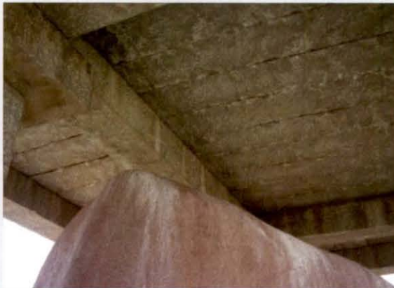
Stains due to water seepage at Ashokan Rock Edict at Nittur, Dharwad
