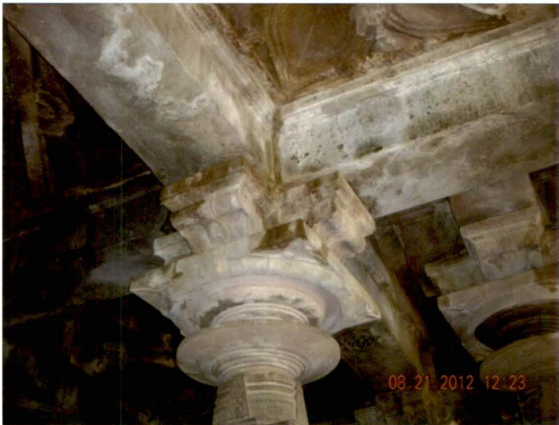
Water seepages in Ramappa Temple after chemical conservation
