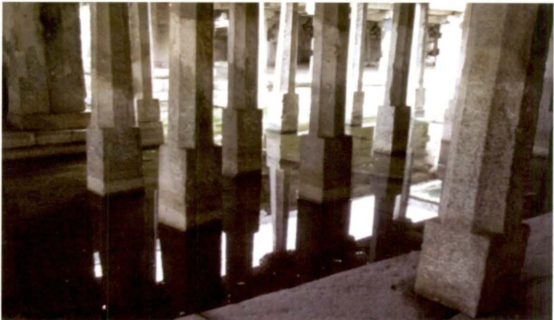
Water logging in Shiva Temple, Hampi, Bengaluru Circle
