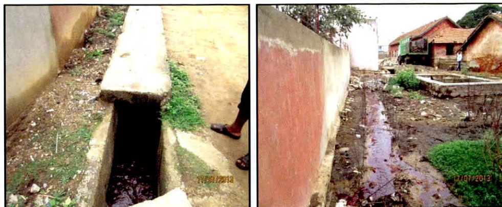
Blood of slaughtered animals flowing through open drain and lying in open at slaughter house, Tannery Road (17 July 2013)
