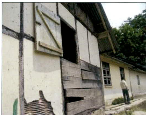
Dilapidated School Building Pakshep JHS, North
