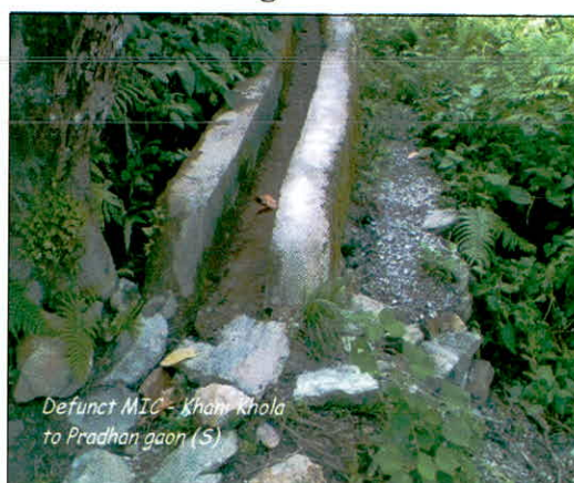
Defunct MIS at Khanikhola to Pradhangaon (S)
