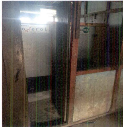
New generator kept in the open without any security, prone to vandalism and vagaries of nature.
