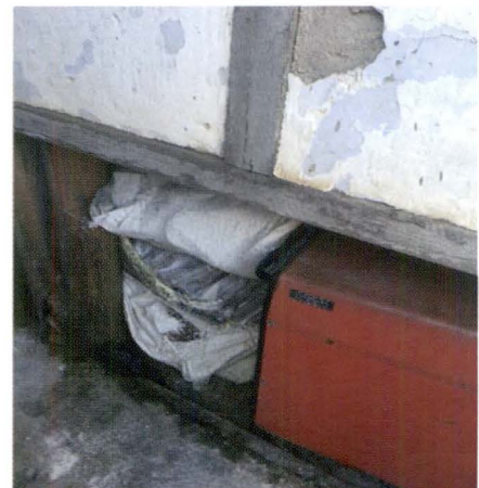
Wall damaged in one of the rooms where Road Permits are kept.
