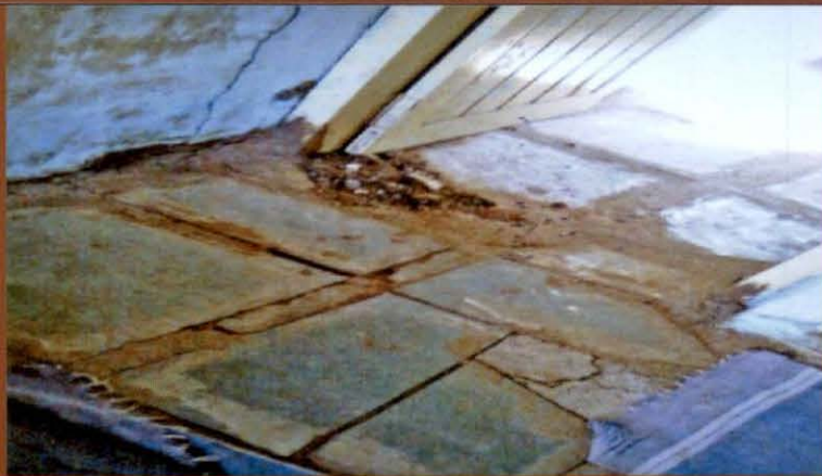
Exhibit 4.7 Poor condition of floor at an Anganwadi Centre building in Gujarat
