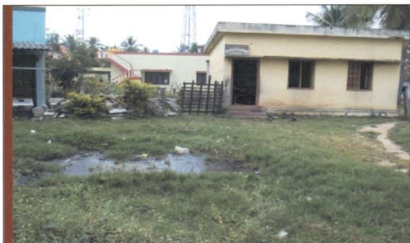
Exhibit 4.15 Unhygienic condition of Anganwadi Centre Ajjampura VI in Karnataka
