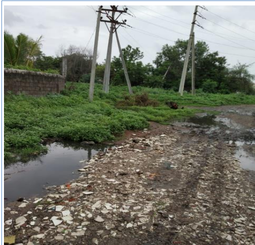
Payakapuram tank without bund/fencing and filled with plants
