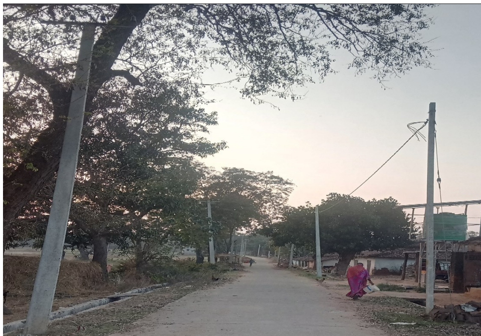
During field visit in Makka village under Ranchi district, it was observed that the TKC did not utilise the existing poles and erected new ones.
