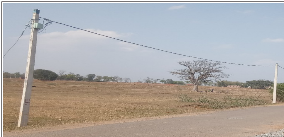
Photograph of SMDB without any connection on a pole at Giridih (photograph taken on 6 March 2020)
