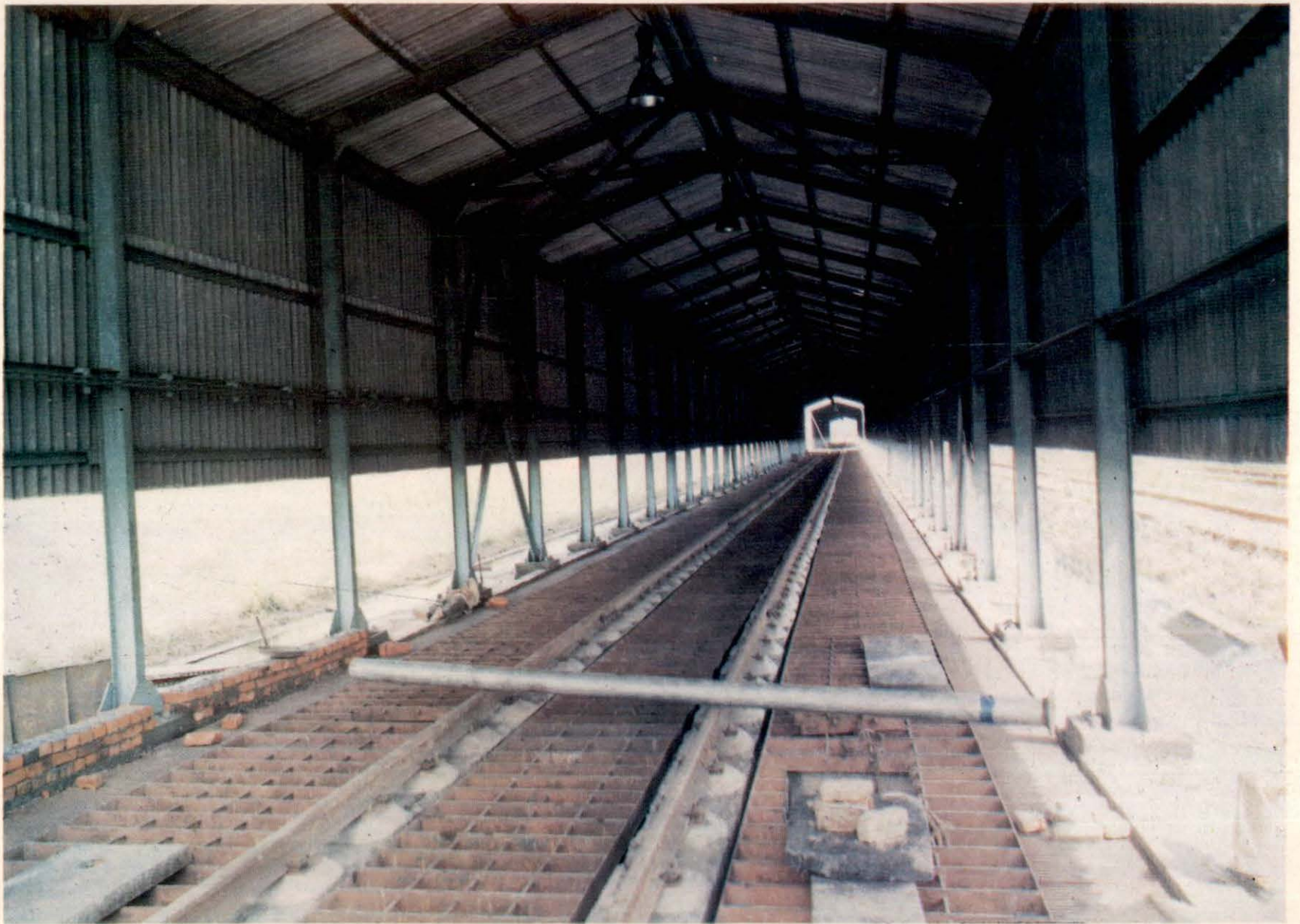
A view of 300 metre long track hopper constructed in May 1992 lying idle (March 1995).
