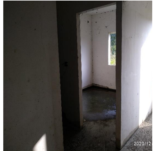
Water clogging in 1BHK flat
