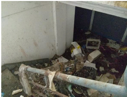
Figure 2.1: Filthy condition of entrance gate of the fish market
