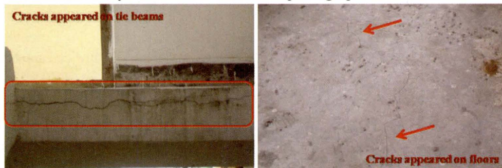
Poor quality of newly constructed Building (Photos taken on 8/6/2011)
