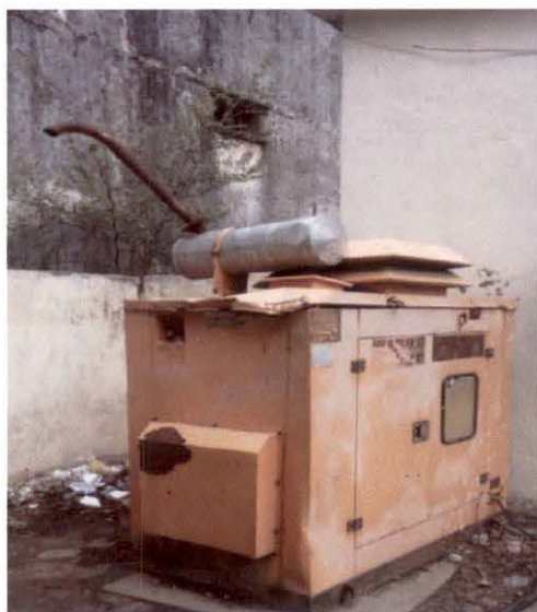
Faulty DG Set at Pop Sanwer, District-Indore
