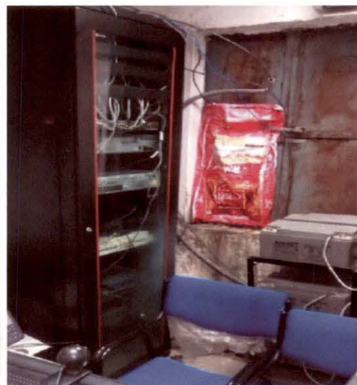
PoP Room at Udaipur, District-Raisen
