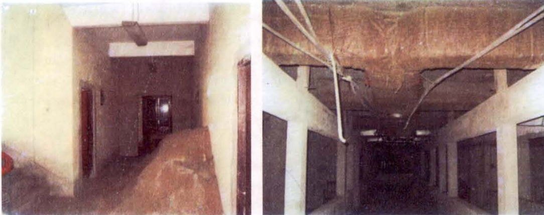
(Photographs of incomplete laboratories of IBV, Khanapara, Guwahati)
