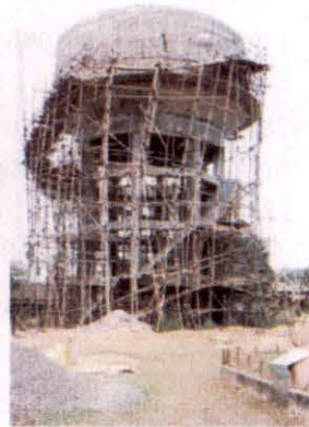
ESR of Dergaon TWSS
