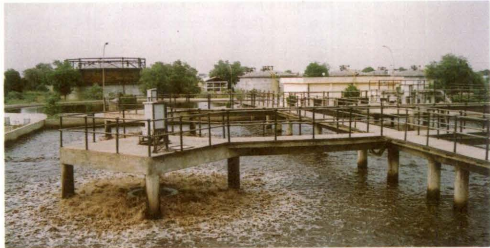
Figure-10: A view of sludge treatment at a sewage treatment plant
