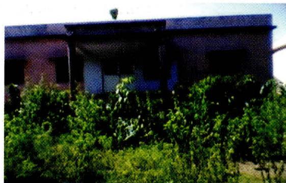
Non-functional CHC building at Boipariguda
