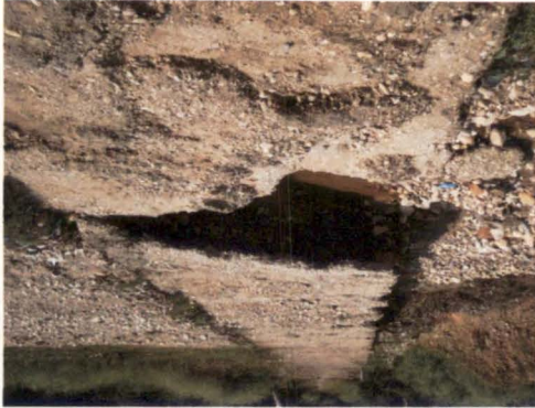
Damaged forest road - Ranipur – Mohand road
