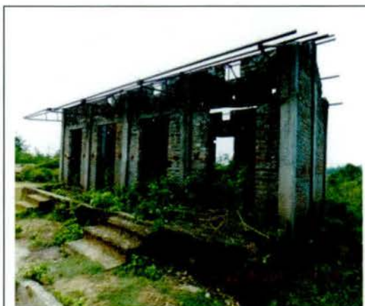
Photograph 4.3.7: Two additional class rooms at Jumercheg Junior Basic (JB) School at Irani Gram Panchayat (GP) under Gournagar Rural Development (RD) Block
