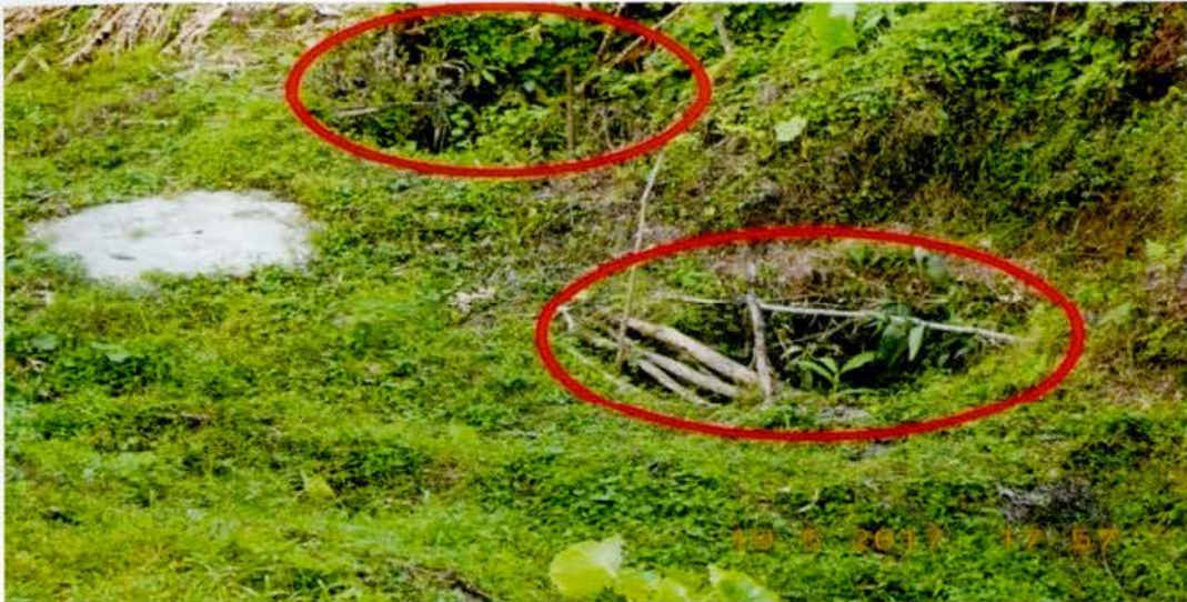
Photograph 4.3.1: Construction of ring well/deep tube well with motor pump (stand by pump) including laying of pipe water storage tanks and iron removal filtration plant at Border Out Post (BOP), Khasiabasti.
