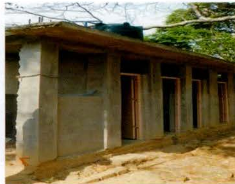
Photograph 4.3.4: Construction of toilet (three unit), bathroom (one unit) with Ordinary Hand Pump (OHP) at Daigyabari
