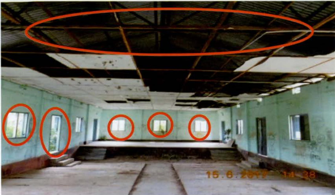
Photograph 4.3.11: Dilapidated condition of the community hall with broken doors, windows and ceiling
