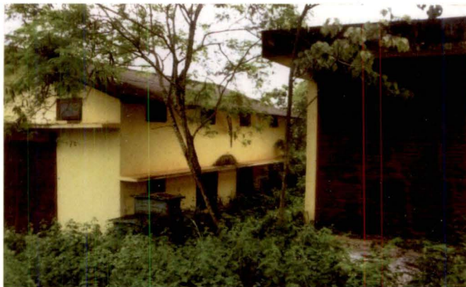
Building of Apparel Park in dilapidated condition
