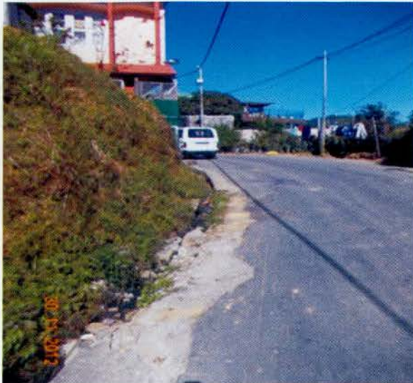
A photograph showing damaged section of the Construction of side drain near Pu Thangdailova (L)'s house to Pi Ruatsangi's house at Chaltlang.
