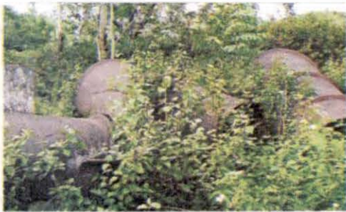
Trifurcation penstock pipes
