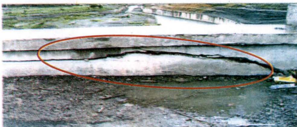
Crack developed in the retaining wall
