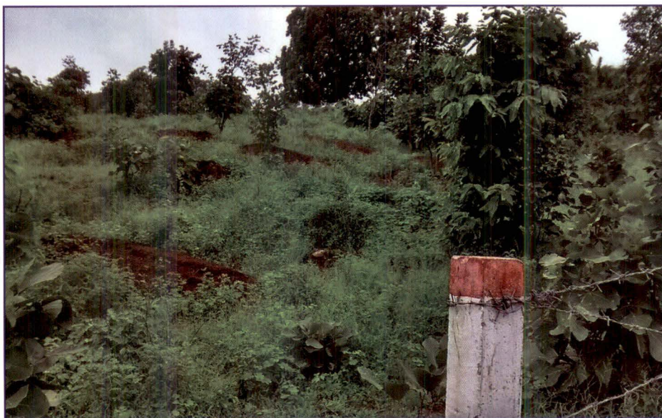
Picture 6 : Contour trench constructed in area with dense vegetation in IWMP-10 of Narmada district (19.08.2014)
