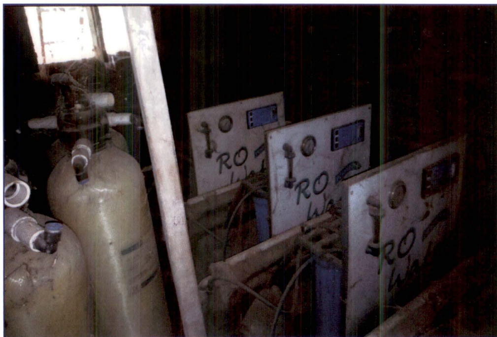
Picture 14 : RO plant lying unutilised at DWDU, Navsari (10.08.2014)
