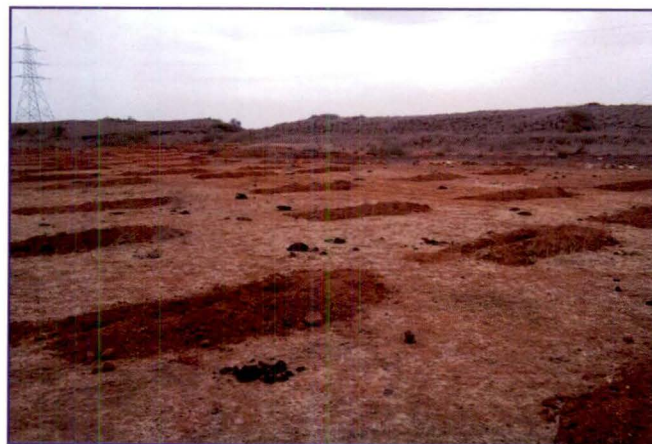
Picture 4 : Contour trench constructed in flat area in IWMP-4 of Kachchh (photo taken at the time of completion of construction work obtained from the records of DWDU)
