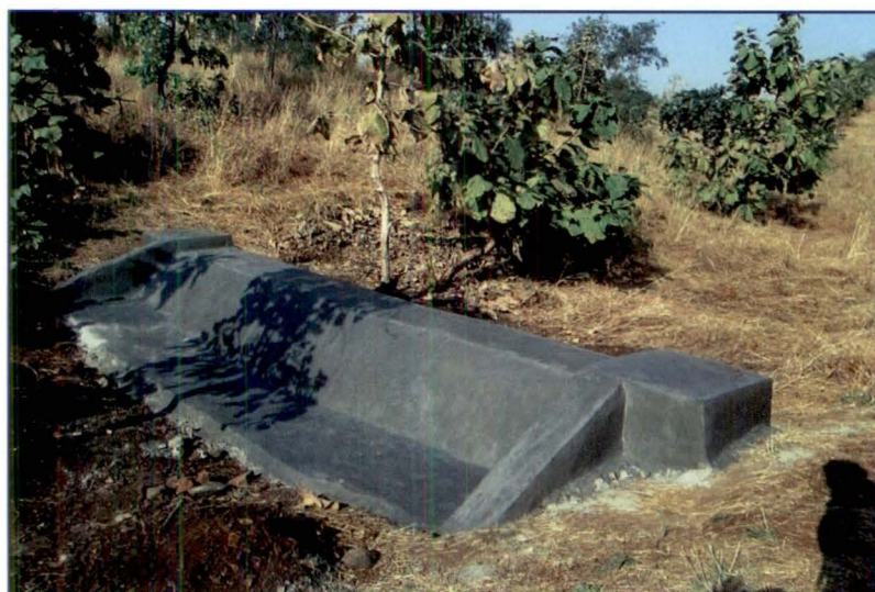
Picture 15: Nala plug without toe wall at IWMP-3, Dahod (02.09.2014)
