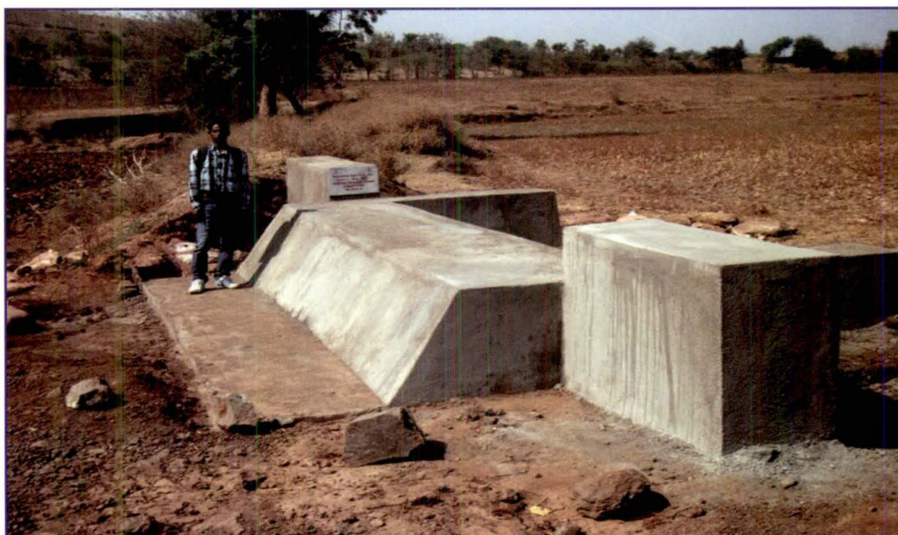
Picture 10: Check wall constructed at Moti-bedvan village in IWMP-3 of Narmada district (19.8.2014)
