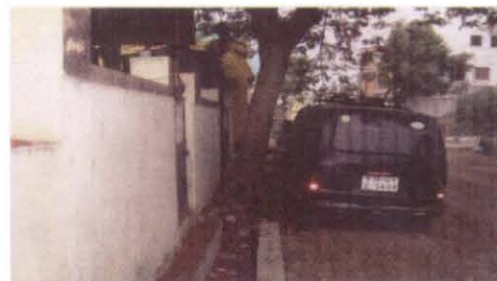
Hindrance of tree in the storm water Drain at Selvapuram
