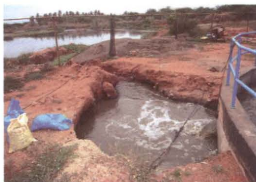
Release of untreated sewage from Avaniapuram Booster Station into open drain
