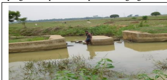
Incomplete Check dam on Sunamuhi Mundakara jore at Tangi Choudwar Block
