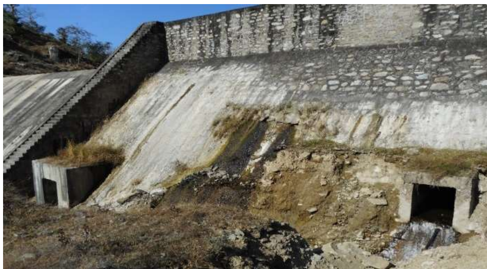
Leakages in the Rohini dam
