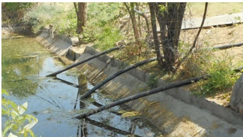
Unauthorised water lifting in NCP as water was taken directly from canals
