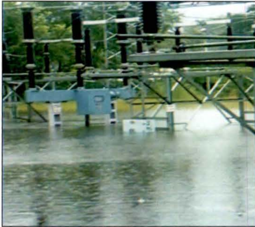
File photo of Switch yard of 132KV SS Bhopatwala Haridwar during flood
