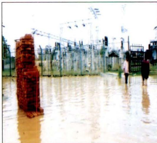
File photo of Switch yard of 132 KV SS at Laksar during flood
