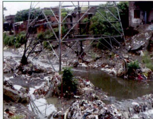
File photo of position of tower with damaged foundation at Bindal River, Dehradun
