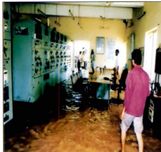
File photo of Control Room of 132 KV SS Laksar during flood
