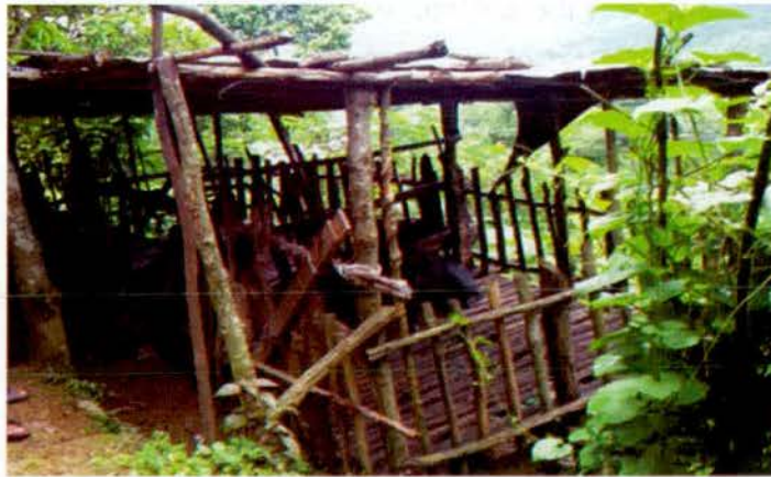
Photograph showing dilapidated pigsty constructed out of first instalment
