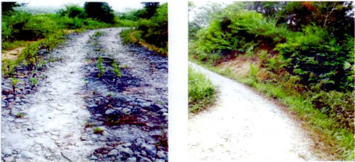
Progress of SMBT Road from Udalthana to New Secretariat as on 4 December 2015
