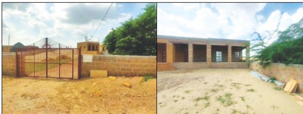
Boundary Wall and Satsang Bhawan , Swangiyani Mandir , GP Myazlar, PS Sam, ZP Jaisalmer (Work ID:2019-20/1826) (Completed: July 2020). Date of Physical verification-28 & 29.9.2021. Work of Boundary wall and Satsang Bhawan at Swangiyani Mandir (Religious Place) was not allowed under BADP.
