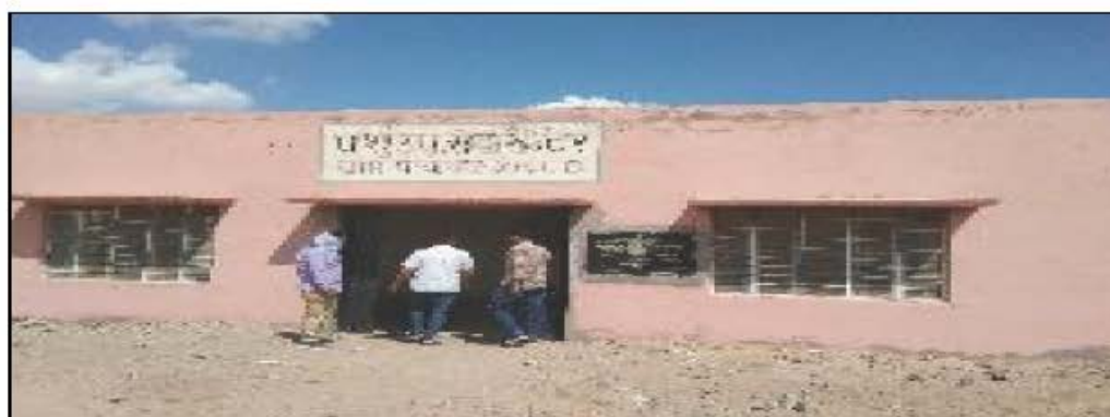
Creation of Animal Sub Center, GP 2 KLD, PS: Khajuwala, ZP: Bikaner (Work ID: 2016-17/12889) (Completed: July 2019). Physical verification during 31.08.2021 to 06.09.2021. Electricity connection not installed and Building was not in use.
