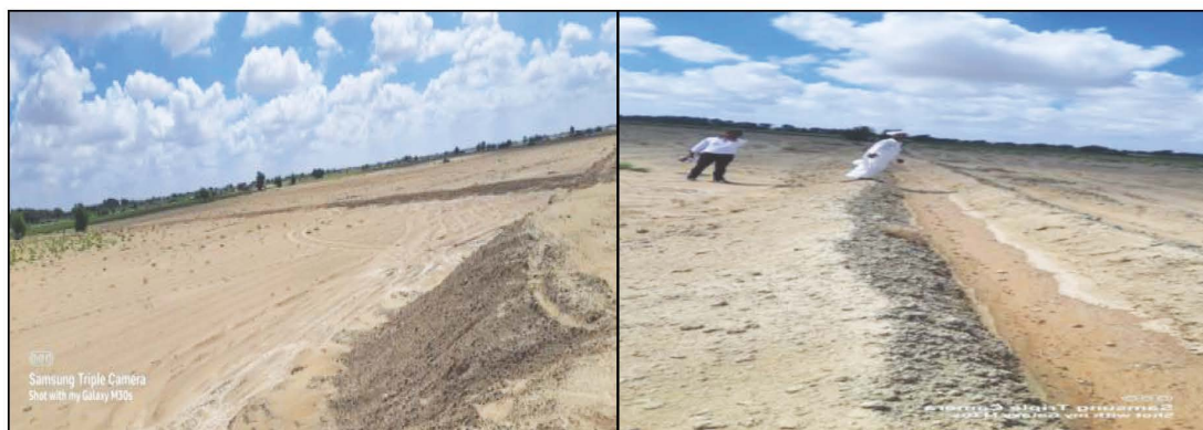
Interlocking Kharanja with nali 1 DTM Khasara no. 227/26 Dittovala, GP: Bandha, PS: Sam, ZP: Jaisalmer (Work ID: 2017-18/31404) (Completed: January 2019). Date of Physical verification-23.09.2021. Assets was not found on the site.
