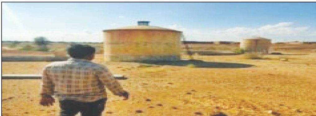
Construction of Ground Level Reservoir (GLR) and Pipeline at Bhawaru Bheel ki Dhani, Punjaram Bheel ki Dhani. (Completed: October 2019). GLR was found to be non-functional.
