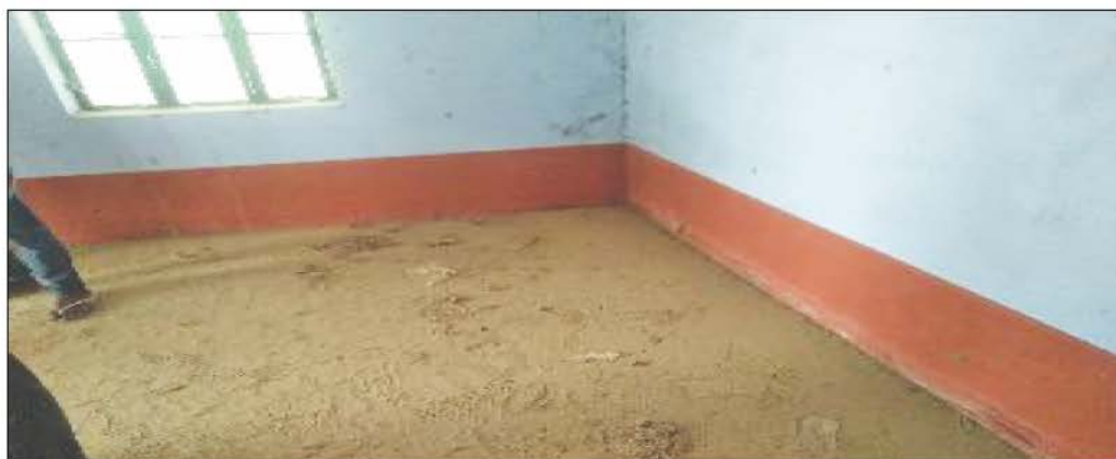
Construction of sub-centre with ANM quarter and maternity home, GP: 20 BD, PS: Khajuwala, ZP: Bikaner (Completed: August 2018). Physical verification during 31.08.2021 to 06.09.2021.
