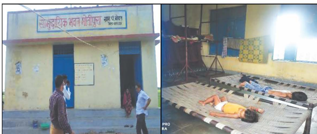
Community Building in village Motipura Ki Jhopadiya, GP Bohat, PS Anta, ZP Baran (Completed: March 2019) being used for personal purpose.
