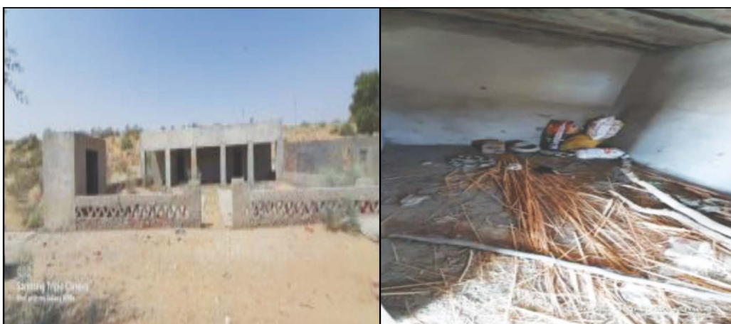
Construction of Community Hall Harnau, GP Harnau, PS: Sam, ZP: Jaisalmer (Work ID: 2017-18/31656) (Completed: November 2018). Date of Physical verification-05.10.2021. Community hall was in bad condition and was not being used for the intended community purpose, it was lying abandoned. There were many Community halls constructed under BADP in the nearby locations.
