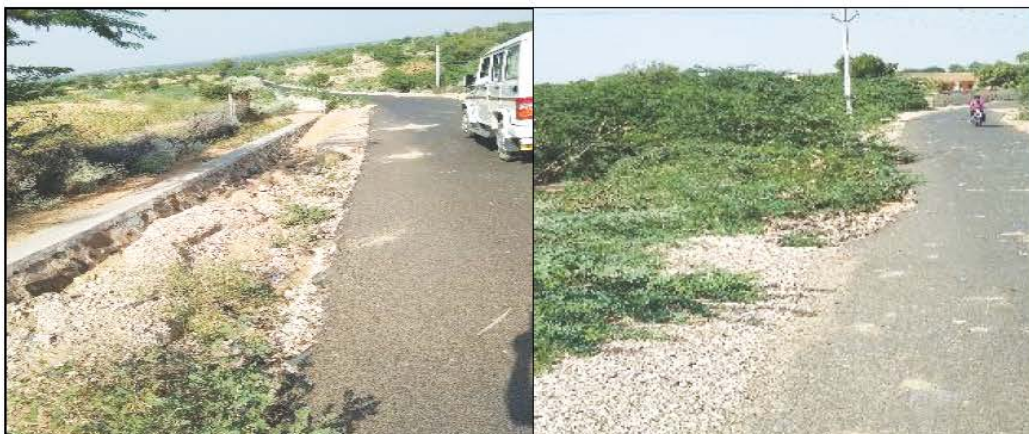
Construction of Bituminous Road Goharka Tala to Bhuromal ki Dhani, GP and PS Chohtan, ZP Barmer (Work ID:2016-17/16713) (Completed: January 2018). Date of Physical Verification 18.10.2021. Road and shoulders was found damaged at various places.
