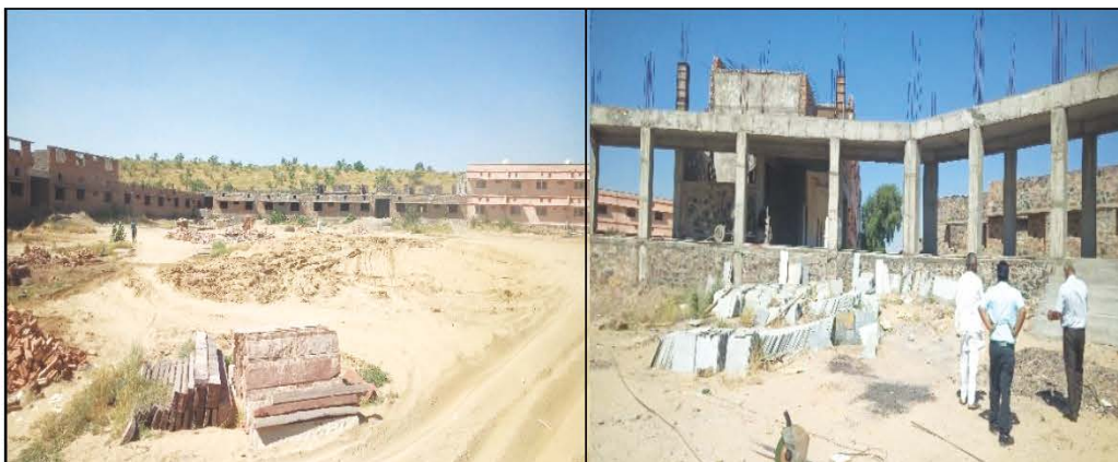
Idle and incomplete Hostel Building (boys) as on 21 October 2021
