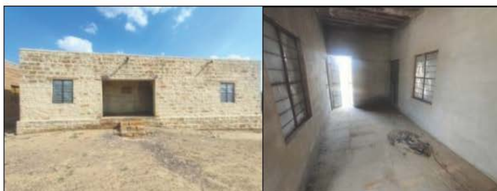
Construction of Residential house for Veterinary Doctor and Staff at Veterinary Hospital, Myazlar, GP: Myazlar, PS: Sam, ZP: Jaisalmer (Work ID: 2018-19/778) (Completed: April 2020). Date of Physical verification- 28-29.09.2021.
