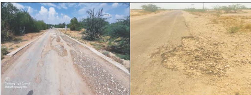
Construction of Bituminous Road from Raghwa to Kalra Kuwa ki Dhani 3 Km, GP Raghwa, PS Sam, ZP Jaisalmer (Work ID:2016-17/14849) (Completed: November 2018). Date of Physical verification-14-09-2021. Road was found in damaged (potholes) condition as maintenance was not being done.
