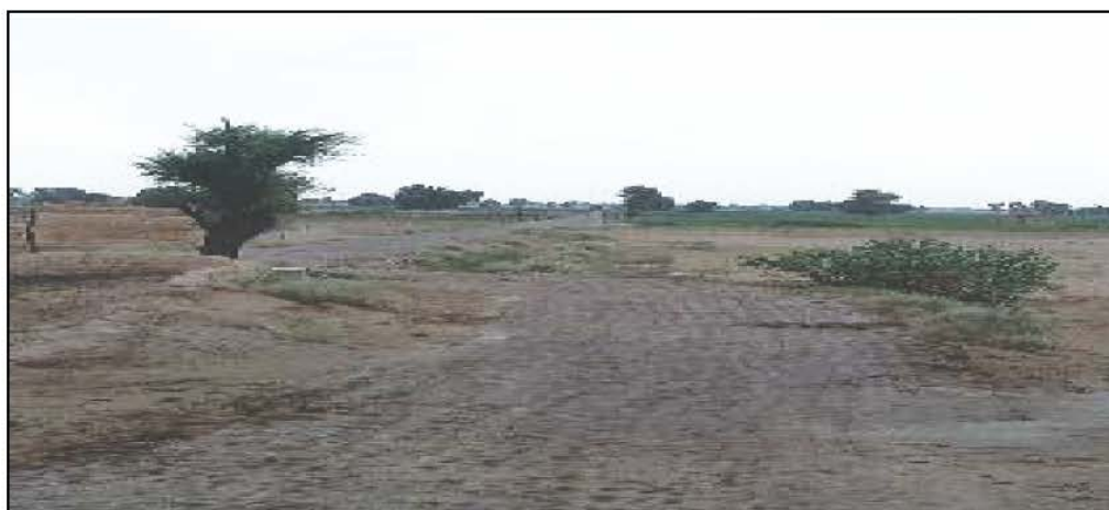
Construction of kharanja road H-minnor to abadi Hishamki, 11 H, GP: 12 H, PS Anupgarh, ZP Sri Ganganagar (Work ID: 2017-18/25139) (Completed: July 2018). Physical Verification during 17.09.2021 to 24.09.2021. Kharanja road was found damaged.
