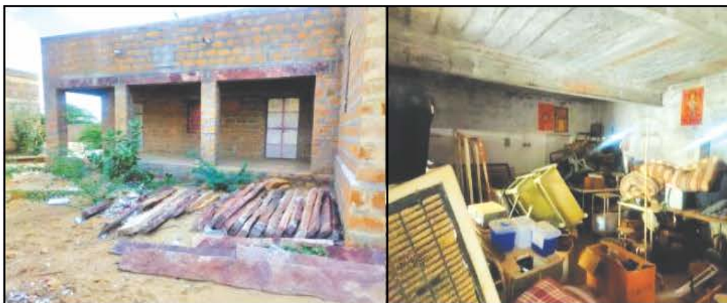
Construction of Labor Room in PHC Myazlar, GP Myazlar, PS Sam, ZP Jaisalmer (Work ID: 2016-17/14871) (Completed: July 2017). Date of Physical verification- 28 and 29.09.2021
