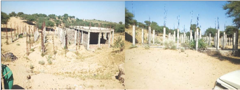
Incomplete work of Polytechnic College building at Jaisindhar Station as on 21 October 2021
