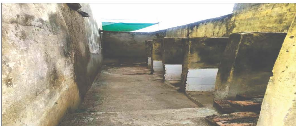
Case 13: Incomplete work of toilet-urinal in Government Senior Secondary School Patiya, GP Patiya PS Kherwara (December 2020).
