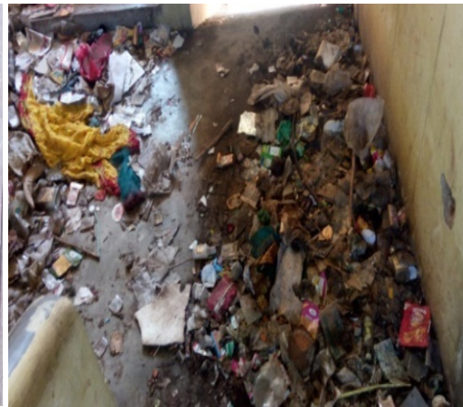
Picture 2.5: Unhygienic waste dumped inside the block
