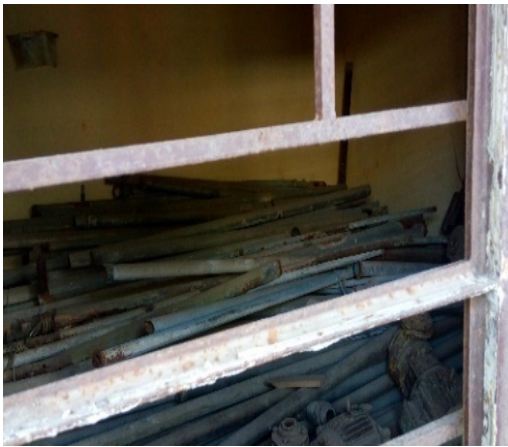
Picture 2.4: Broken window and waste material dumped
