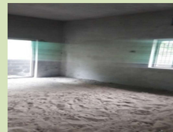
Figure-3.9: Incomplete Mahila Sangam building (07 July 2018)
