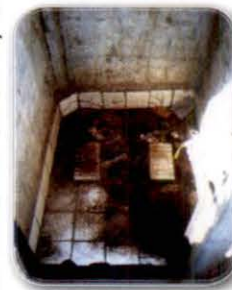
Picture 3 Toilet seat in Kamboi PS, Dahod (02.04.2013)
