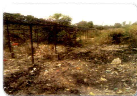
Picture 15 Incomplete VCP at Dholka NP, Ahmedabad District (10.04.2013)
