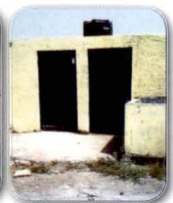
Picture 4 Toilet in Chavaj PS, Bharuch without water connection (29.05.2013)
